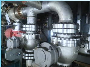
Sinopec Great Wall Energy Chemical (Ningxia) Co., Ltd. Chilling Water Pump Shut-off Valve May.2018
