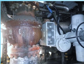
Shaanxi Shenmu Chemical Industry Co., Ltd. Chilling Water Pump Shut-off Valve Oct.2013
