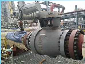
Ningxia Baofeng Energy Synthetic Device Electric valve for water, coal and gas inlet conversion area May.2020
