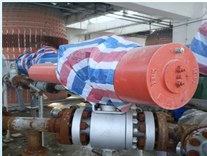
CNSG Anhui Hong Sifang Co., Ltd. Coal Slurry Circulation Pipeline Reflux Regulating Valve 5.4MPa Hooking up interlock in 2020
