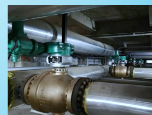
Inner Mongolia Rongxin Chemical Co., Ltd. Chilling Water Pump Shut-off Valve in 2019
