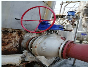
Shaanxi Jincheng Coal Industry Group Tianxi Coal-to-Oil Bureau Flash Tank Outlet Shut-off Valve May.2020
