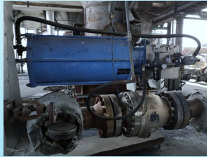
Yankuang Guohong Chemical Co., Ltd. Black Water Grey Water Shut-off Valve Aug.2015
