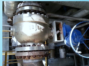
Sinopec Qilu Petrochemical Bureau Chilling Water Pump Shut-off Valve Feb.2013
