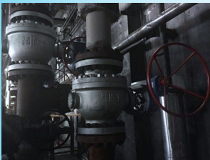
Ningxia Baofeng Energy Chilling Water Pump Shut-off Valve Nov.2016
