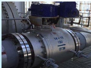
CNOOC Huizhou Coal-to-Hydrogen Production Unit Sulfur recovery jacket insulation valve Waste heat boiler sulfur process gas July.2018
