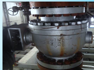
Yanzhou Coal Yulin Energy Chemical Co., Ltd. Chilling Water Pump Shut-off Valve June.2013
