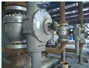
Henan Jindadi Chemical Co., Ltd. Electro-hydraulic Linkage Chilling Water Pump Shut-off Valve Feb.2019
