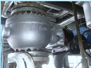
Inner Mongolia Xinneng Energy Co., Ltd. Electric Chilling Water Pump Shut-off Valve May.2013
