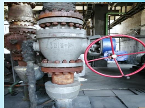
Henan Jinkai Chemical Investment Holding Group Co., Ltd. Chilling Water Pump Shut-off Valve Aug.2019
