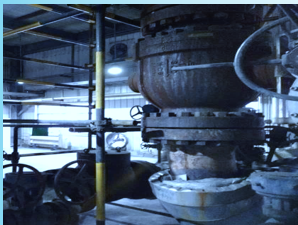
Shenhua Baotou Coal Chemical Industry Co., Ltd. Electric Chilling Water Pump Shut-off Valve Sept.2014
