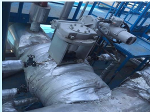
Sinopec Jinan Bureau Delayed Coking Tower Top Vent Isolation Valve Replaces VELAN Bellows Ball Valve Sept.2014
