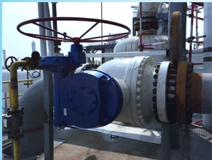
Wanhua Chemical Group Co.,Ltd. (Ningbo) Syngas Vent Isolation Valve Sept.2015
