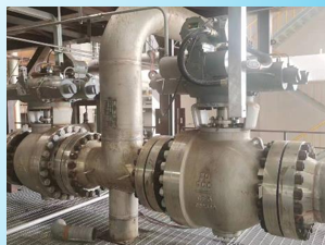
Shandong Hualu Hengsheng Group Co. (Jinzhou) Electro-hydraulic Linkage Chilling Water Pump Shut-off Valve Dec.2022
