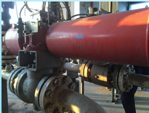
Wanhua Chemical Group Co.,Ltd. Coal Slurry Circulation Pipeline Reflux Regulating Valve 5.4MPa Hooking up interlock Sept.2014
