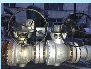
Yankuang Xinjiang Energy Chemical Co., Ltd. Gasification Black Water Switching Double Valve June.2014
