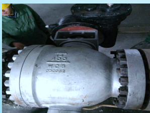
Xinjiang Xinlianxin Energy Chemical Co., Ltd. Chilling Water Pump Shut-off Valve Sept.2014
