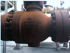
Nanjing Chengzhi Clean Energy Co., Ltd., Chilling Water Pump Shut-off Valve May.2012
