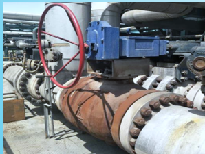
Shandong Hualu-Hengsheng Group Co.,Ltd. Chilling Water Pump Shut-off Valve June.2015
