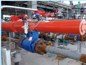
Shandong Hualu-Hengsheng Group Co.,Ltd. Coal Slurry Circulation Pipeline Reflux Regulating Valve 5.4MPa Hooking up interlock Sept.2017
