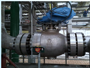
Ningxia Baofeng Energy Synthetic Device Manual valve for Desulfurization Tank Inlet and Outlet May.2020
