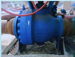
GDDG Syngas Compressor Inlet and Outlet Isolation Valves in 2021
