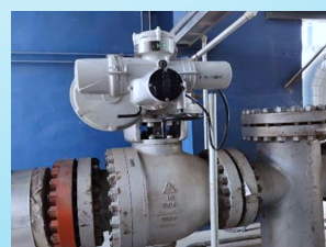
Shandong Jincheng Petroleum Group Chilling Water Pump Shut-off Valve in 2019
