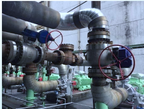
Sinopec Nanjing Branch Company 8.7MPa Chilling Water Pump Shut-off Valve Dec.2016
