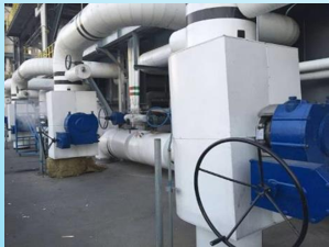
Wanhua Chemical Group Co.,Ltd. Chilling Water Pump Shut-off Valve Sept.2015
