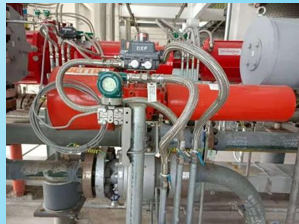
Huineng Group Coal Slurry Circulation Pipeline Reflux Regulating Valve 5.4MPa Hooking up interlock in 2021
