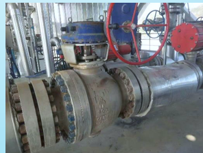
Shaanxi Yanchang Petroleum Yan'an Energy&Chemical Co.,Ltd. High Pressure Black and Gray Water Shut-off Valve Aug.2018
