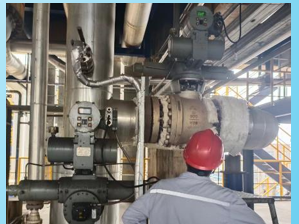
Zhejiang Baling Hengyi Caprolactam Co., Ltd. Electro-hydraulic Linkage Chilling Water Pump Shut-off Valve Dec.2021
