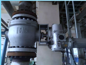
Guangxi Huayi Energy Chemical Co., Ltd. Chilling Water Pump Shut-off Valve in 2021
