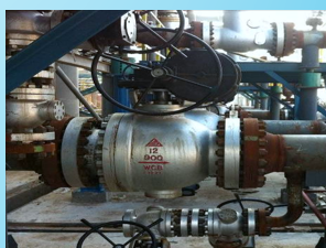
Ordos Jinchengtai Chemical Co., Ltd. Chilling Water Pump Shut-off Valve Feb.2013
