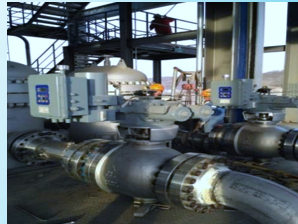
Shaanxi Yanchang Petroleum Yan'an Energy&Chemical Co.,Ltd. Electro-hydraulic Linkage Chilling Water Pump Shut-off Valve Sept.2018
